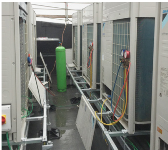
Main cooling system
