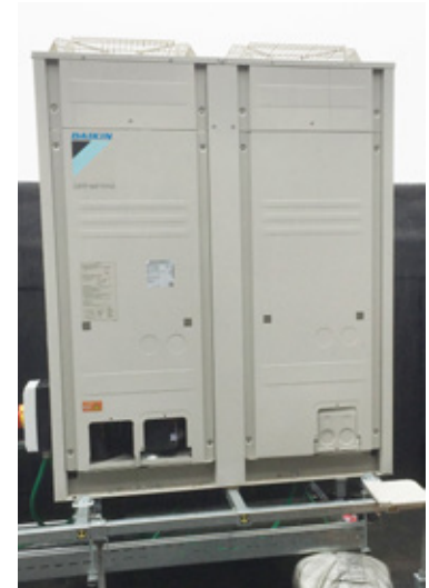
Standby heat pump
